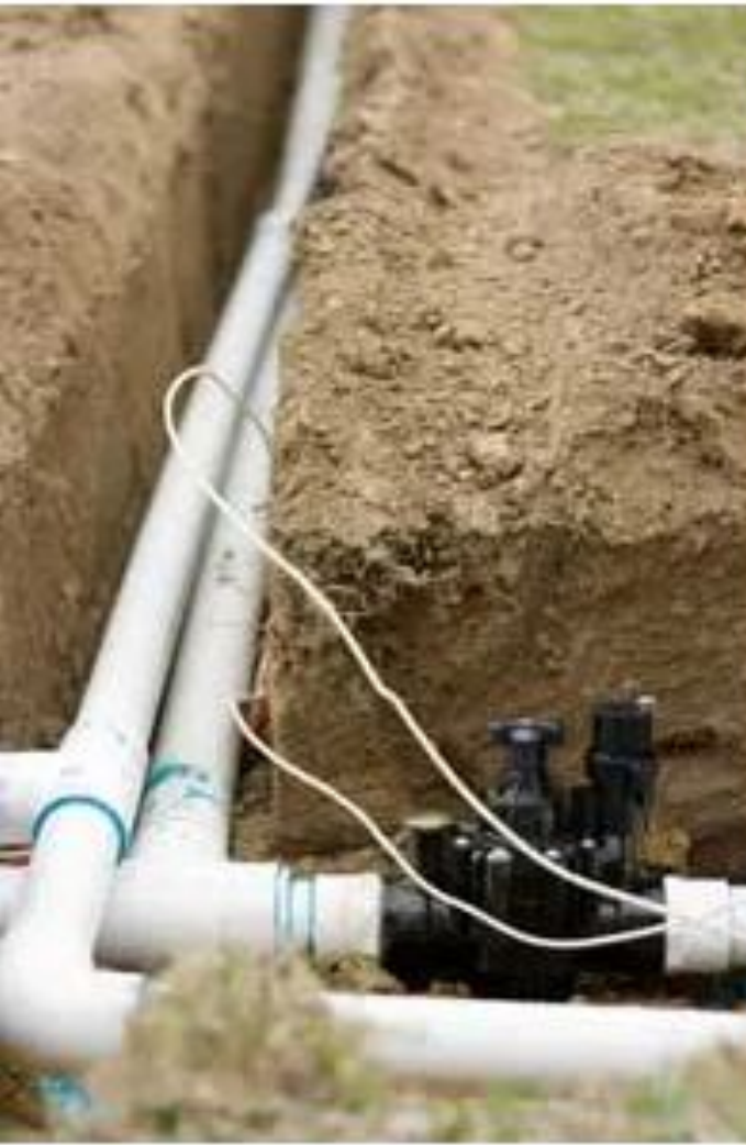
Irrigation & Livestock Pipeline
